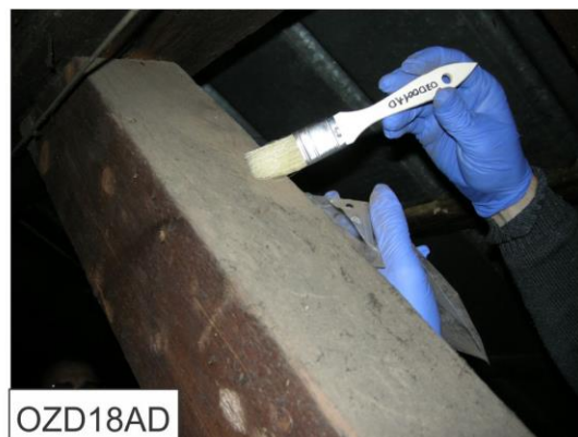
3. Dust (sample) on the beam
